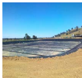
A 14ML covered anaerobic lagoon at Bungowannah. A 6,000 sow 'breeder only' piggery 2012 = 4,000 to 9,000 cows (grazing herd) = 700 to 1,200 cows (freestall)
